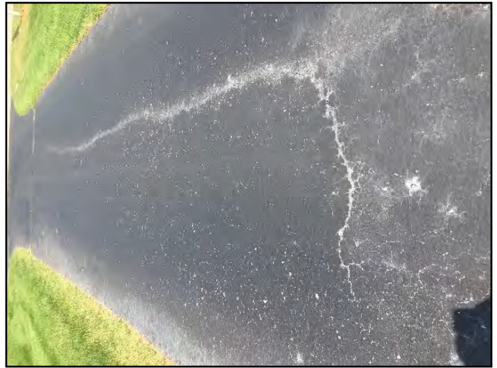
24. Cracked or damaged surfaces
