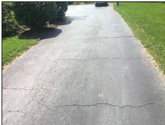
25. Cracked or damaged surfaces
