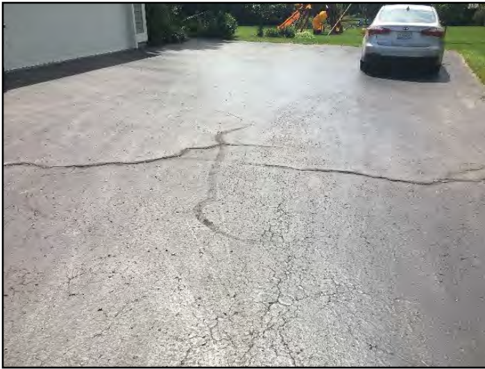
23. Cracked or damaged surfaces
